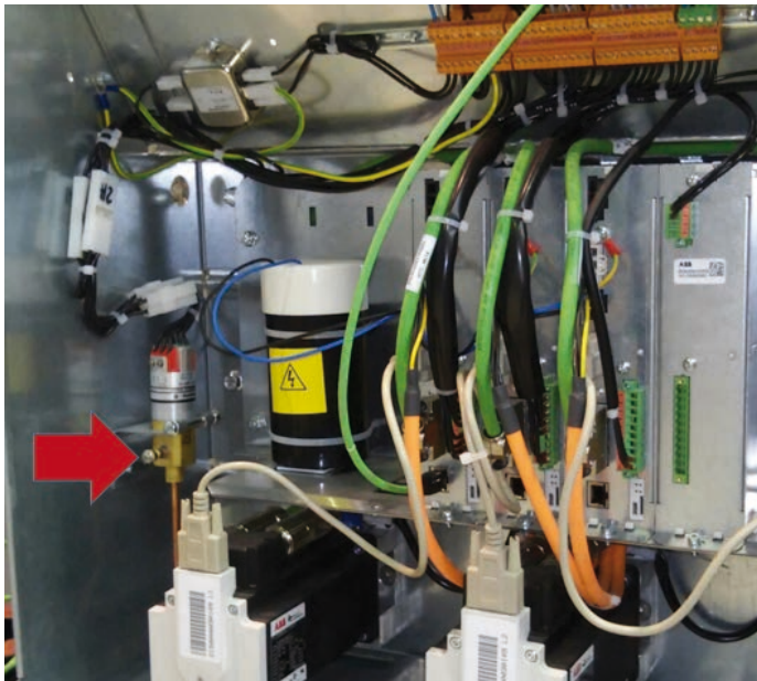
Figure 23. DS1 pressure sensor with its charging valve
